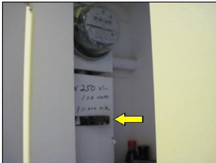
Main disconnect switch for 5089 rear cupboard
