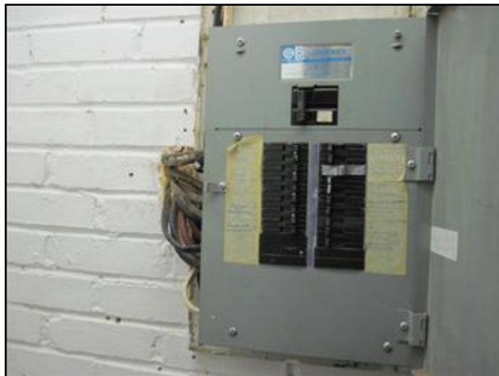
Distribution panel for unit 5093
