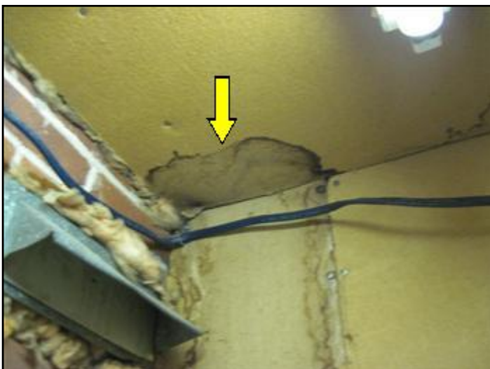
Water stain utility room 5093
