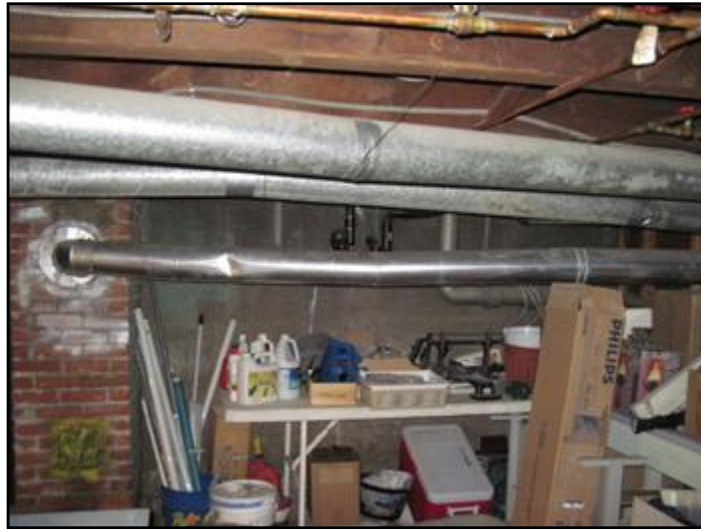
Vent slope questionable
