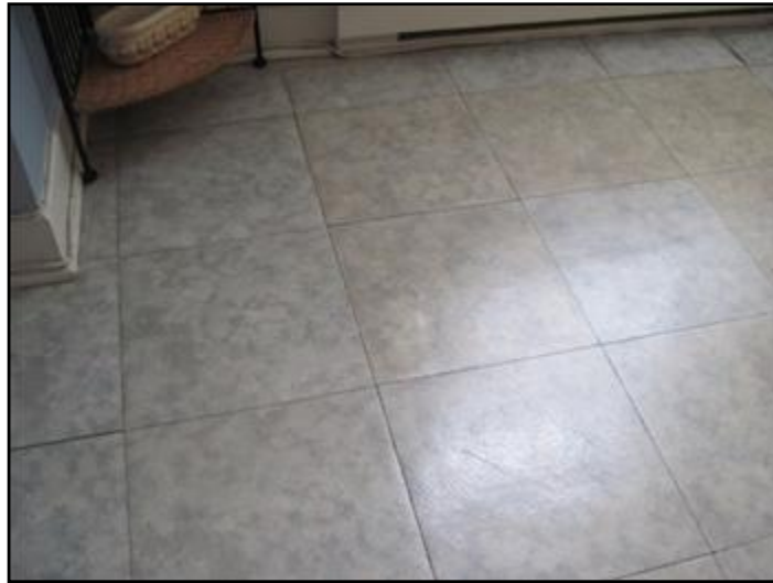
Discoloration of flooring tiles visible
