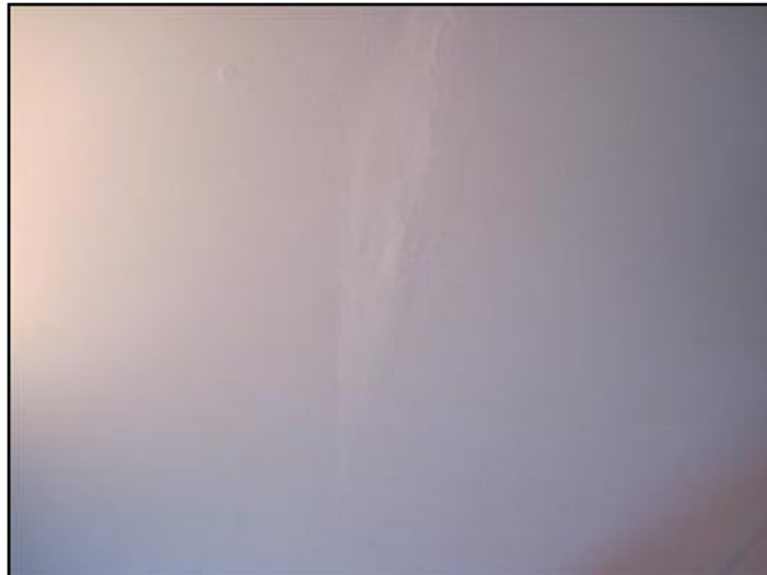
Crack visible in kitchen ceiling
