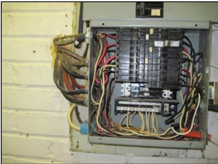
View inside the distribution panel for 5091
