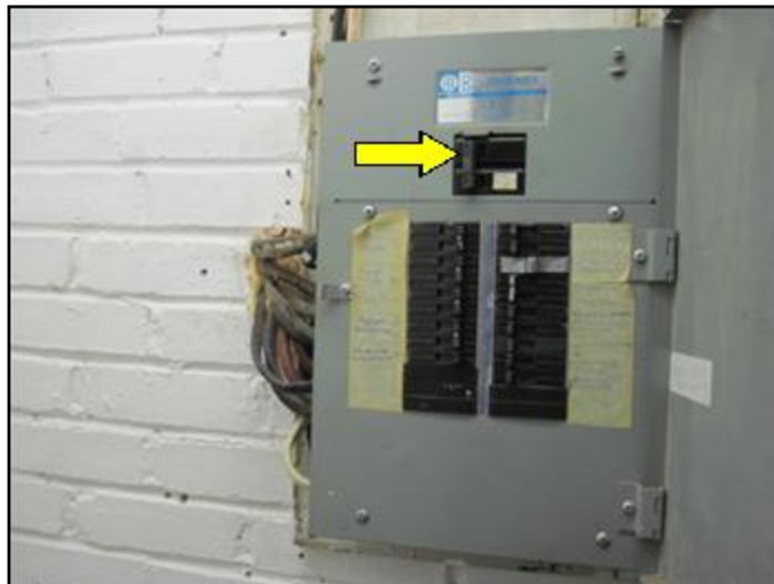
Main electrical switch for 5091
