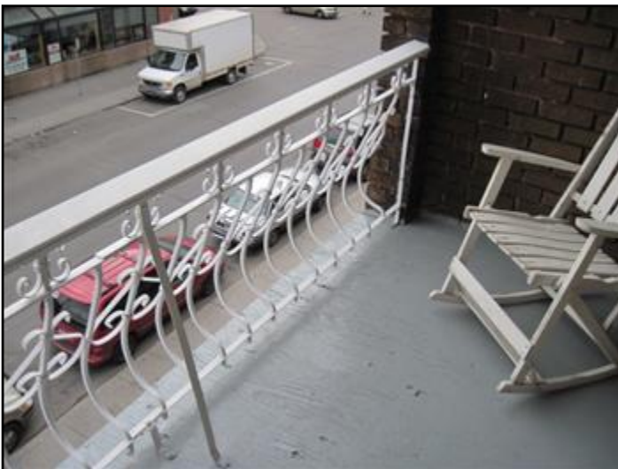
Front balcony guardrail's too low
