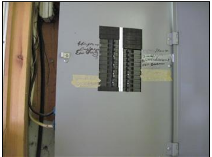
Distribution panel for 5093
