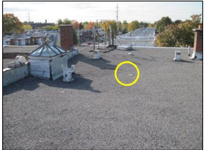
Location of blister on roof
