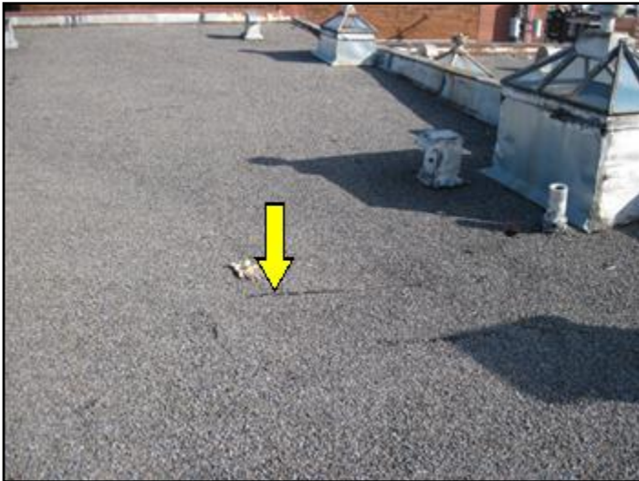
Location of blister on roof
