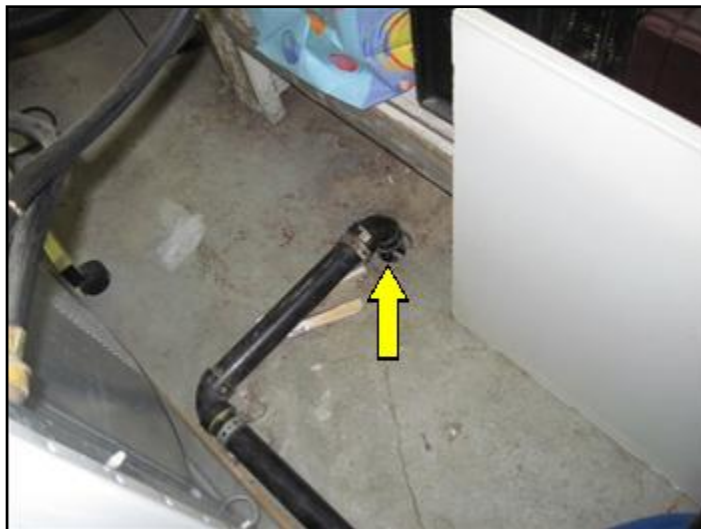
Laundry tub drain pipe over floor drain
