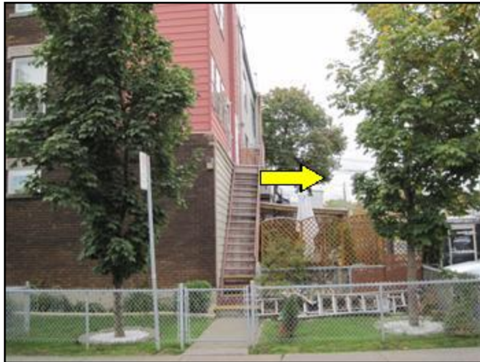
Rear staircase leaning to the right
