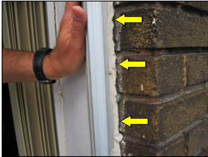
Caulking has shrunk leaving an open gap
