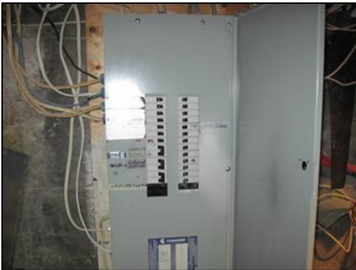
Distribution panel for unit 5089 in basement
