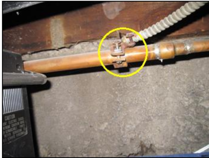
Ground connection to water pipe in basement
