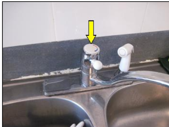
Loose control arm
