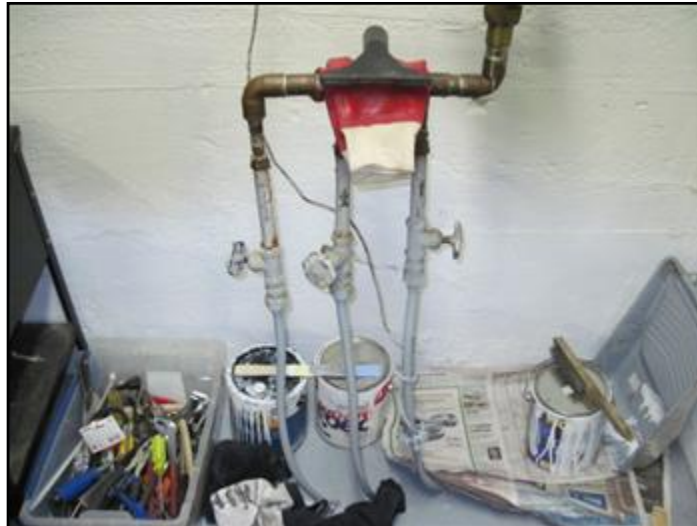
Water main valves in basement
