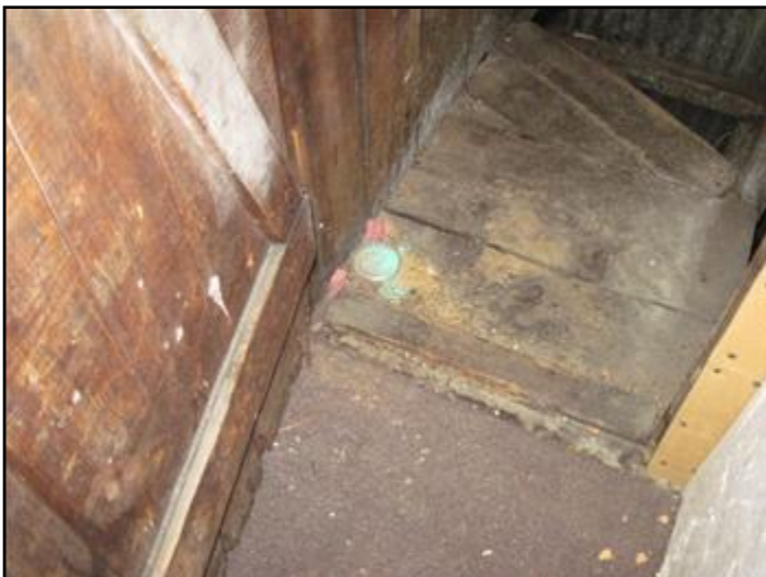
Rodent bait trap utility room 5093
