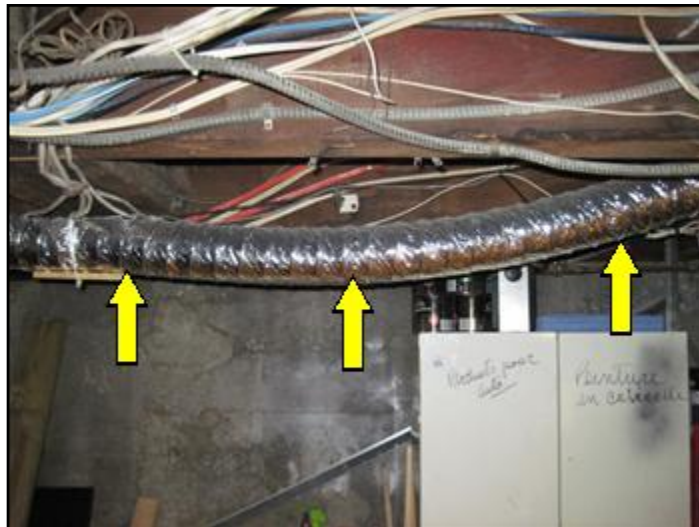
Flexible pipe for dryer in basement
