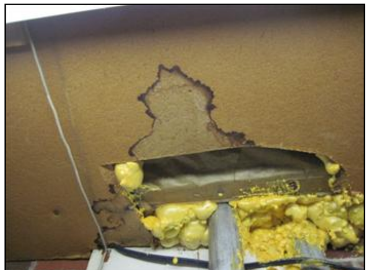
Water stain utility room 5093
