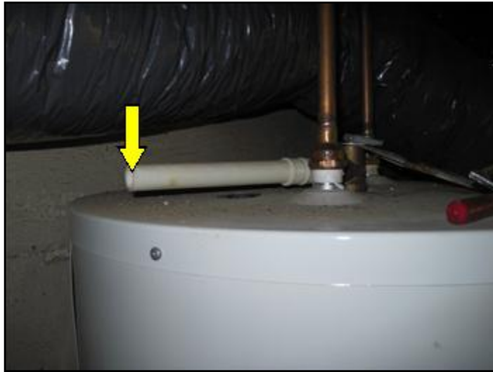
Discharge tube too short
