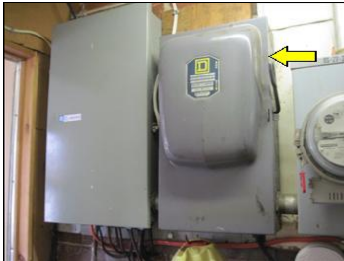
Main electrical switch for 5093
