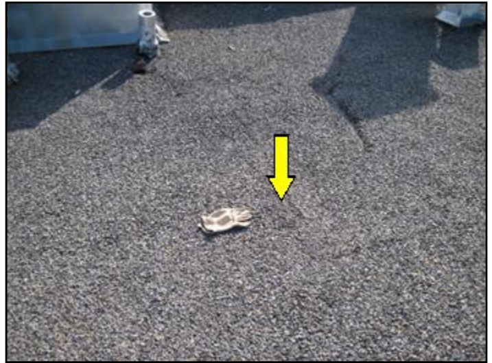
Location of blister on roof
