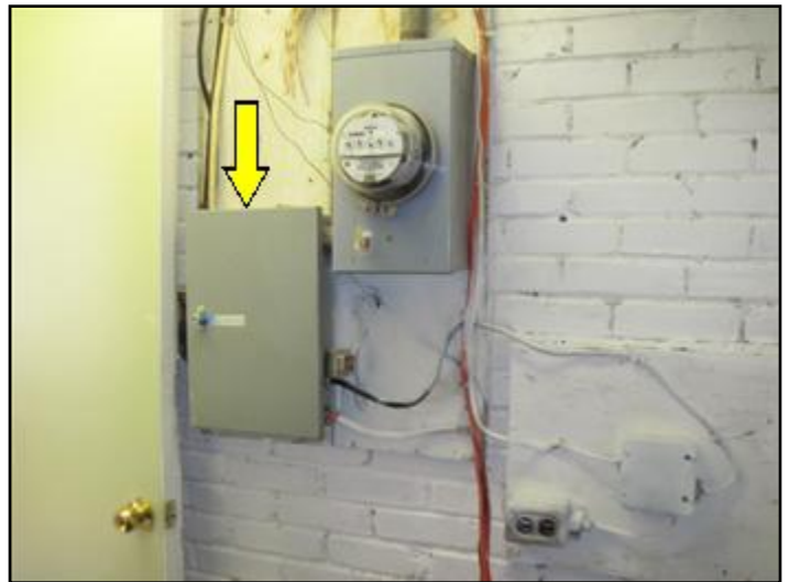
Distribution panel and main switch for 5091
