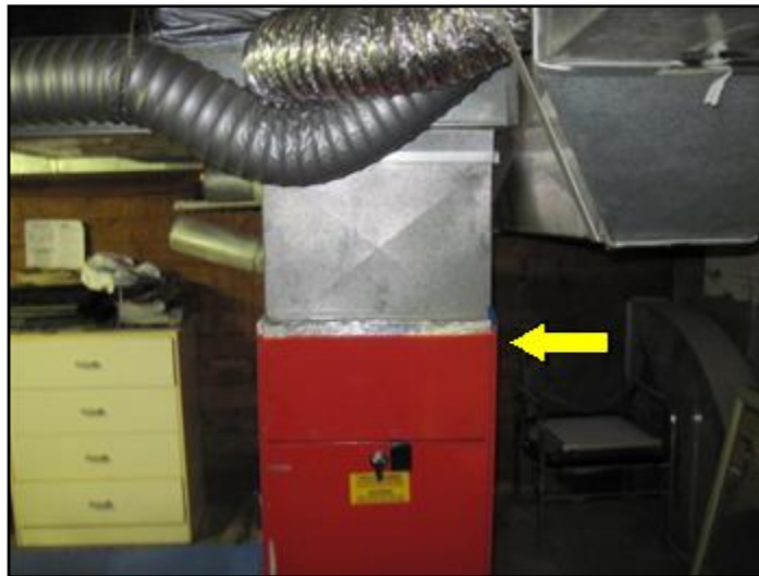
Gas fired forced air furnace for 5089
