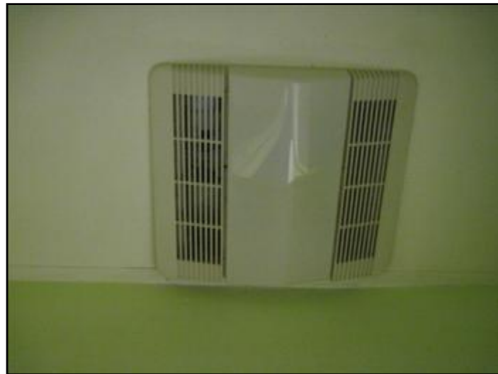
Bathroom fan not functional in 5089
