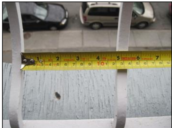
Spacing between bars exceeds 4"
