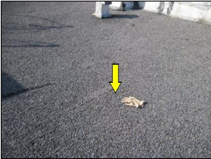
Location of blister on roof
